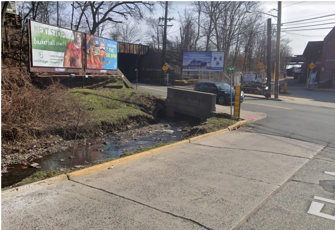
Photo 2: Undersized culvert underneath River Road.
