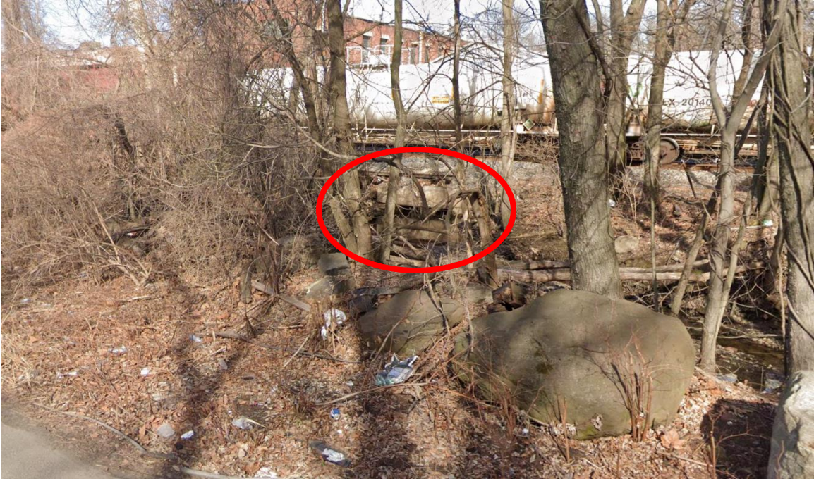
Photo 11: Existing undersized culvert seen in the background below the NYSW railroad tracks.
